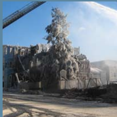
BEFORE Last winter a fire devastated a block of homes being built by Habitat for Humanity in Lawrence.
