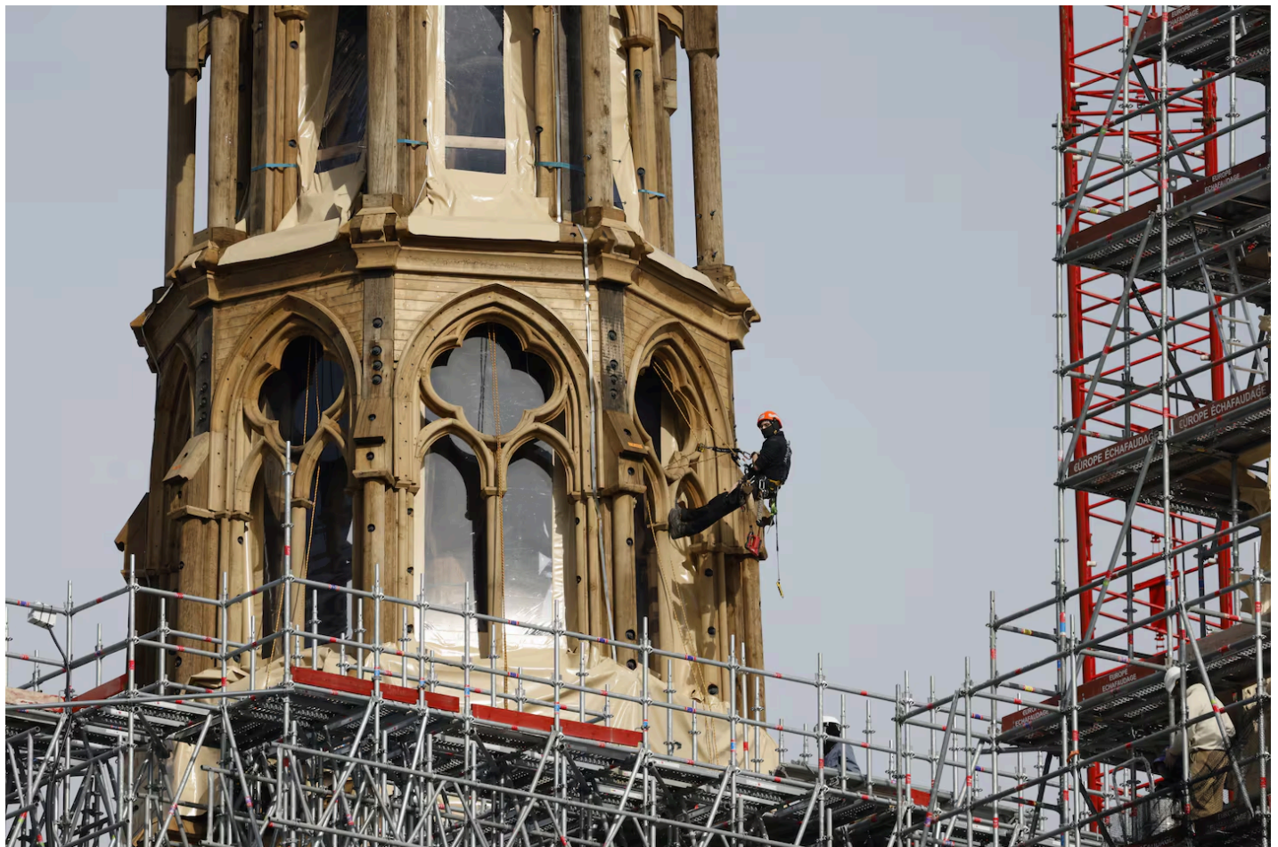
A worker operated on the reconstruction of Notre Dame Cathedral's new wooden spire in Paris on March 14. LUDOVIC MARIN/AFP VIA GETTY IMAGES
